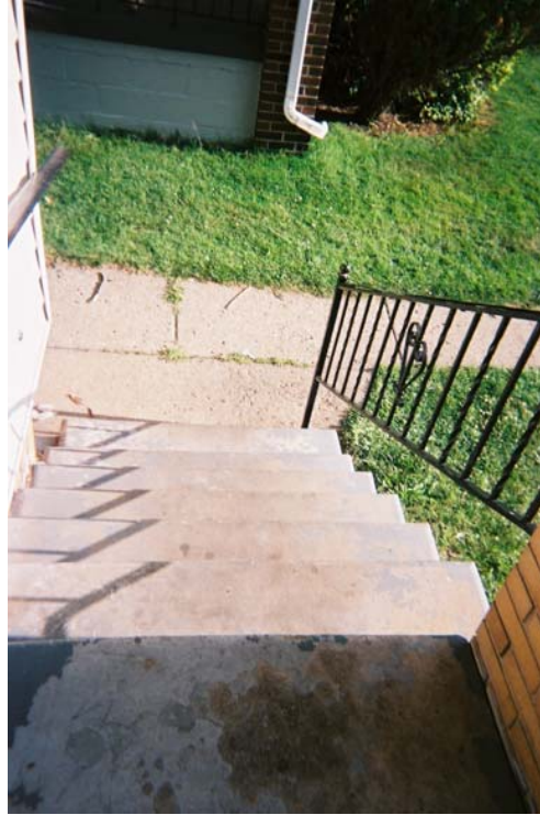
Figure 24. Challenges with chronic pain - Stairs and unsafe railing
